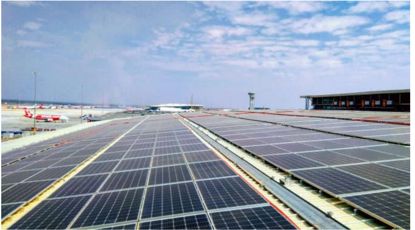
Solar installation at Bengaluru Airport Pic credit: bialairport.com
